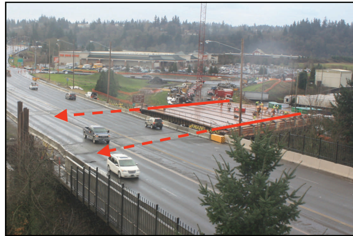
The new bridge, currently under construction on the west side of the highway, will slide into its permanent position.
